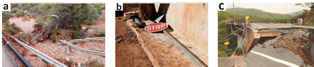
Fig. 4. Damage on infrastructure due to floods and earthquakes, including (a) damaged road fences, (b) broken road signs (Diakakis et al. 2020), and (c) damage to the Tawarayama bridge (Aye et al. 2018).
